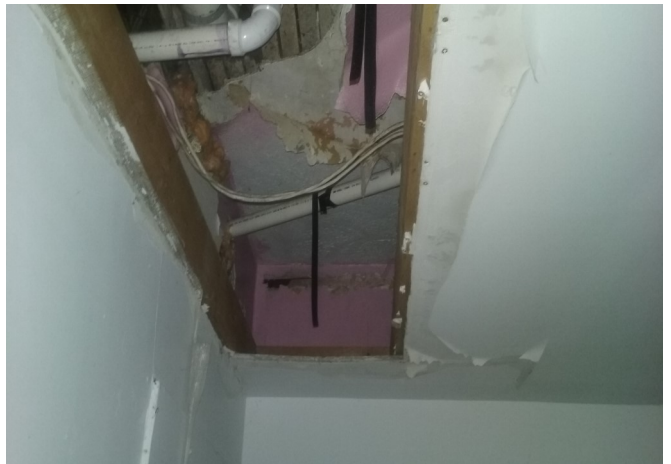
Ceiling damage needs repaired.
