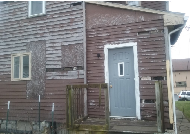
External damage needs repaired.
