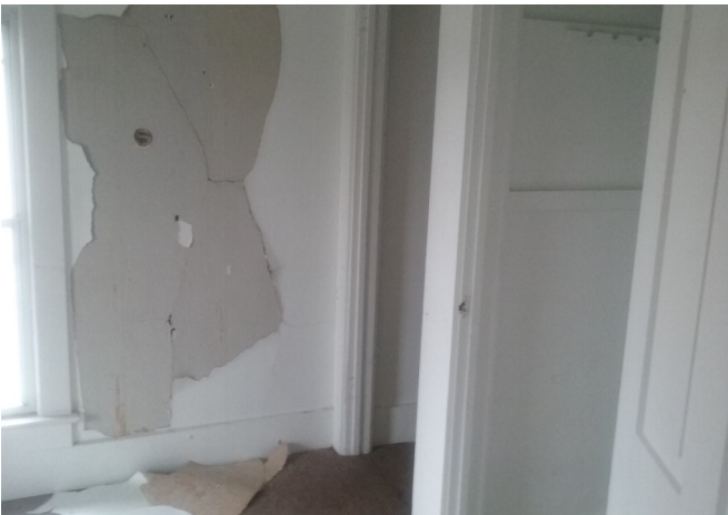
Interior walls throughout need repaired.
